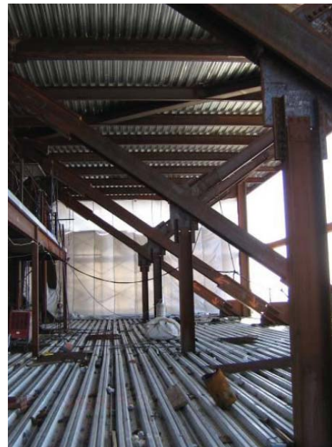
Figure 7: Outrigger bracing on mechanical floor, courtesy of Thornton Tomasetti
